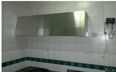
New extraction hood installed in the soup kitchen
